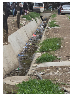
ii. A new drainage near Government complex, clogged with litter
